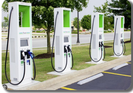
EV Charging Stations (Incentivized through SCE)
