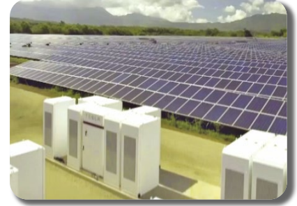
Solar Photovoltaic + Battery Storage
